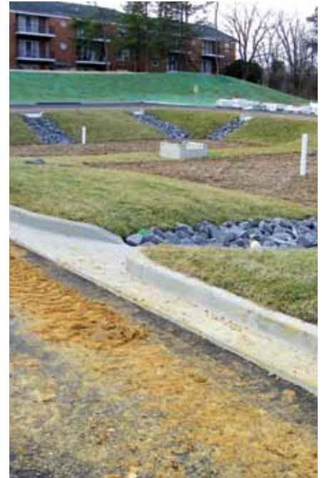
An urban stormwater management system is installed at the Lexington Park Volunteer Rescue Squad in St. Mary's County.
