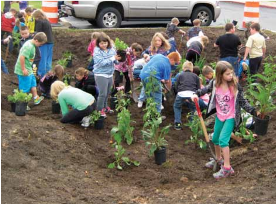
In 2014, the Allegany SCD spearheaded the installation of rain gardens and a bioswale to capture stormwater runoff at a local elementary school.
