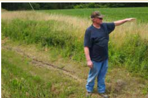
Practicing What We Preach — John Swaine, III, chairman of the Talbot Soil Conservation District, installs an innovative two-stage ditch on his property to reduce runoff entering a creek near his home. The pilot practice is the first of its kind in Maryland. If successful, it could be duplicated throughout the Eastern Shore.
