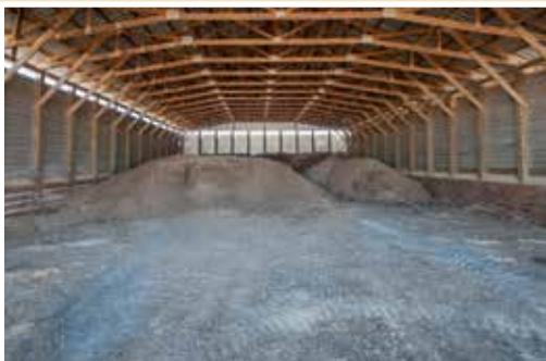
Helping Farmers Comply with Their Nutrient Management Plans — This poultry waste storage structure protects water resources on the Eastern Shore.
