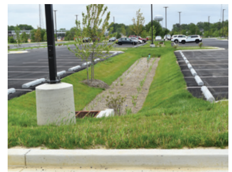
A stormwater management structure catches and treats parking lot runoff at the new Leonardtown Library in St. Mary's County.
